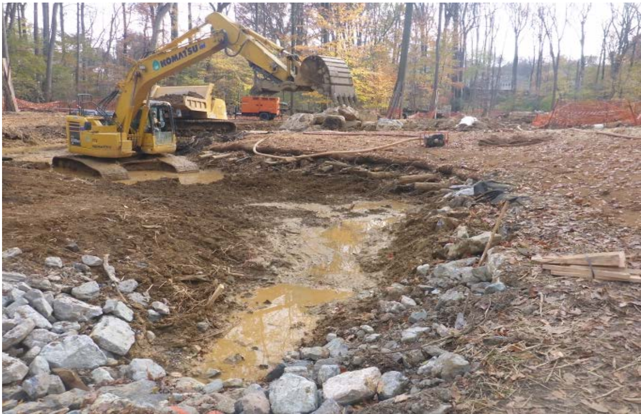
Fig. 1. A recent stream construction project at Upper Watts Branch Forest Preserve, City of Rockville, Maryland. Notice that the existing stream was completely destroyed to create an artificial floodplain by clearing the forested valley and raising the channel with tons of fill (sediment), tree trunks, and boulders. Photo by City of Rockville.
