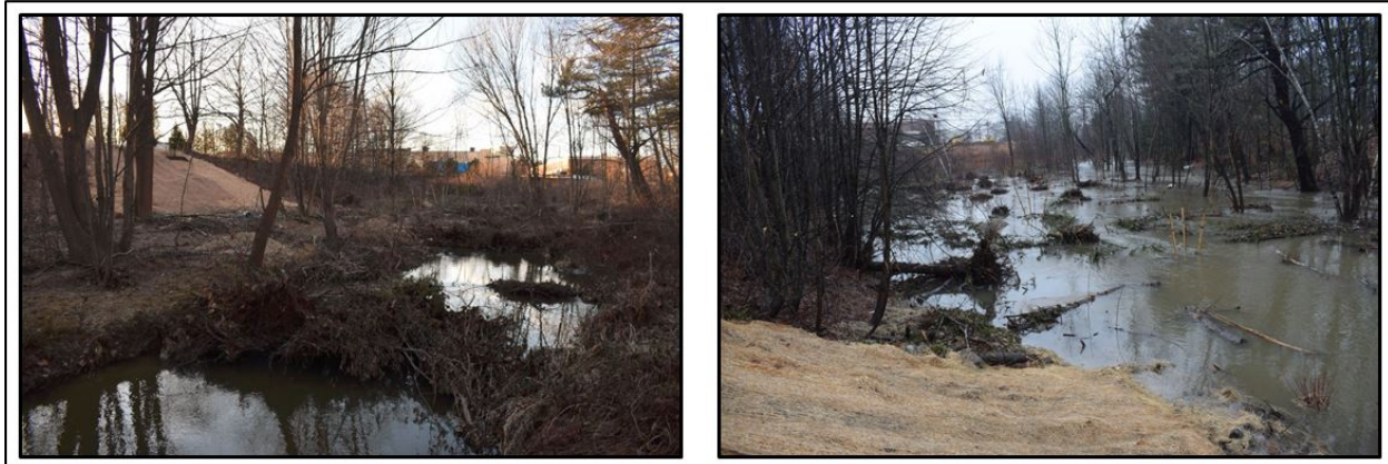
Figure 1. Log jams (left) constructed on an incised portion of Long Creek in South Portland, ME to restore floodplain flow (right).
