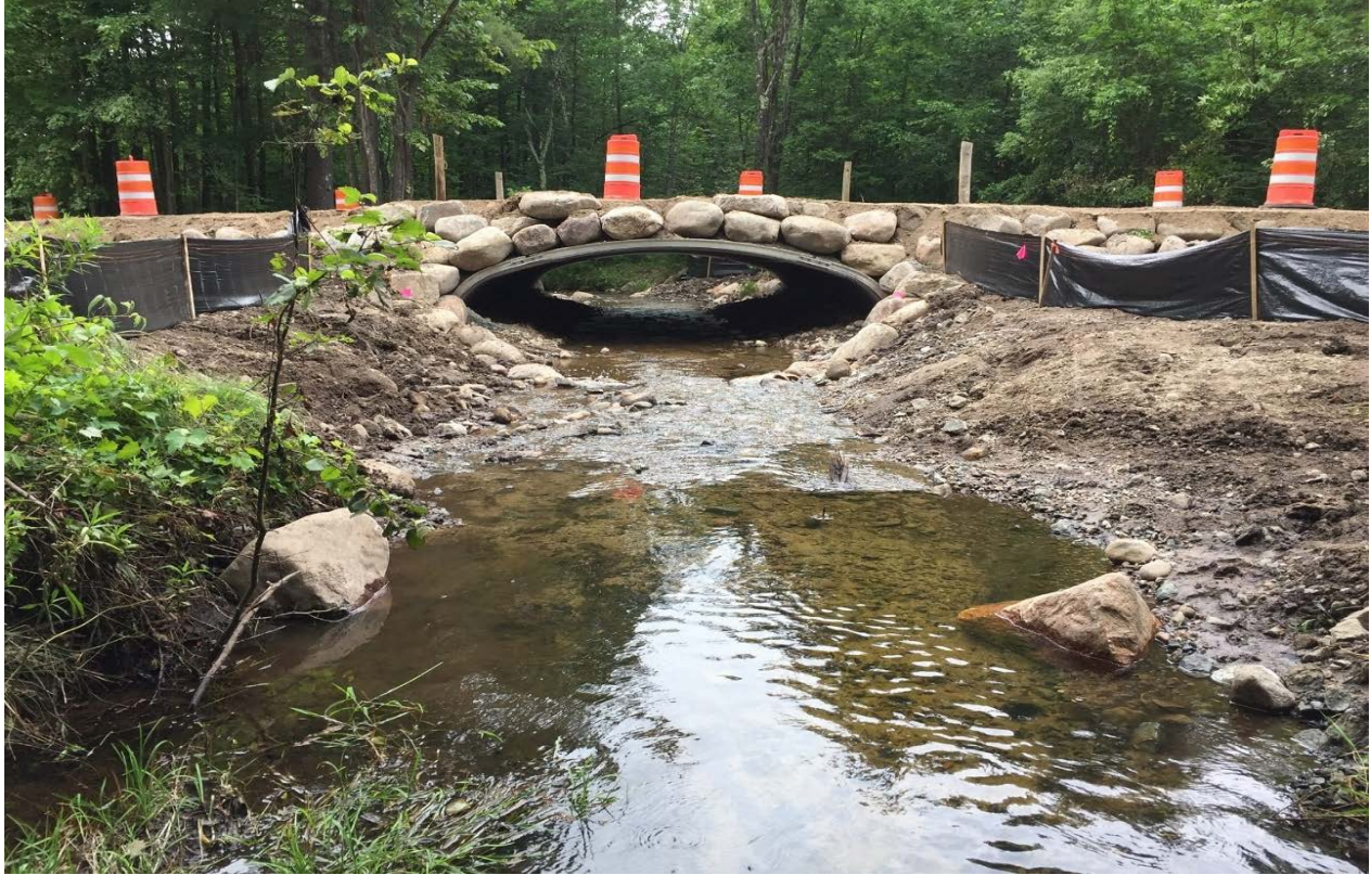
Fig. 4. An example of an attractive, effective, and flood-resilient road-stream crossing and redesign that reconnects the stream to its floodplain. The project is part of the Climate-Ready Culvert Initiative in the Ausable River watershed. Photo courtesy the Adirondack Almanack.
