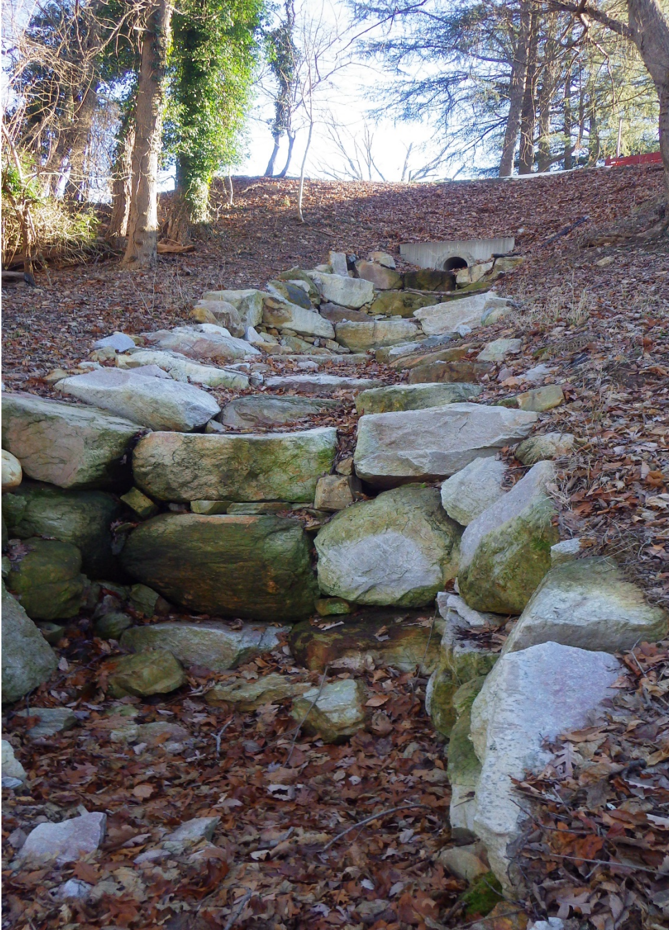
Fig. 1. A high-quality, joint National Park Service-Department of Defense project to restore a stormwater blowout on a steep slope in old-growth Mesic Mixed Hardwood Forest at Arlington Woods bordering Arlington National Cemetery and Arlington House in Arlington County, Virginia. Natural-to-the-site quartzite sandstone boulders were carefully installed along the blowout, forming a series of plunge steps, and no trees were harmed or removed for the project. Infestations of English Ivy and other non-native invasive plants cover much of the forest, as they do at the Hollin Hills sites, though are slowly being removed here. The effects of sheetflow runoff from impervious surface into the site are also much the same as observed at Goodman Park. Also notice that because the forest community was retained, the site is not planted with a myriad of inappropriate species. Photo by R.H. Simmons.
