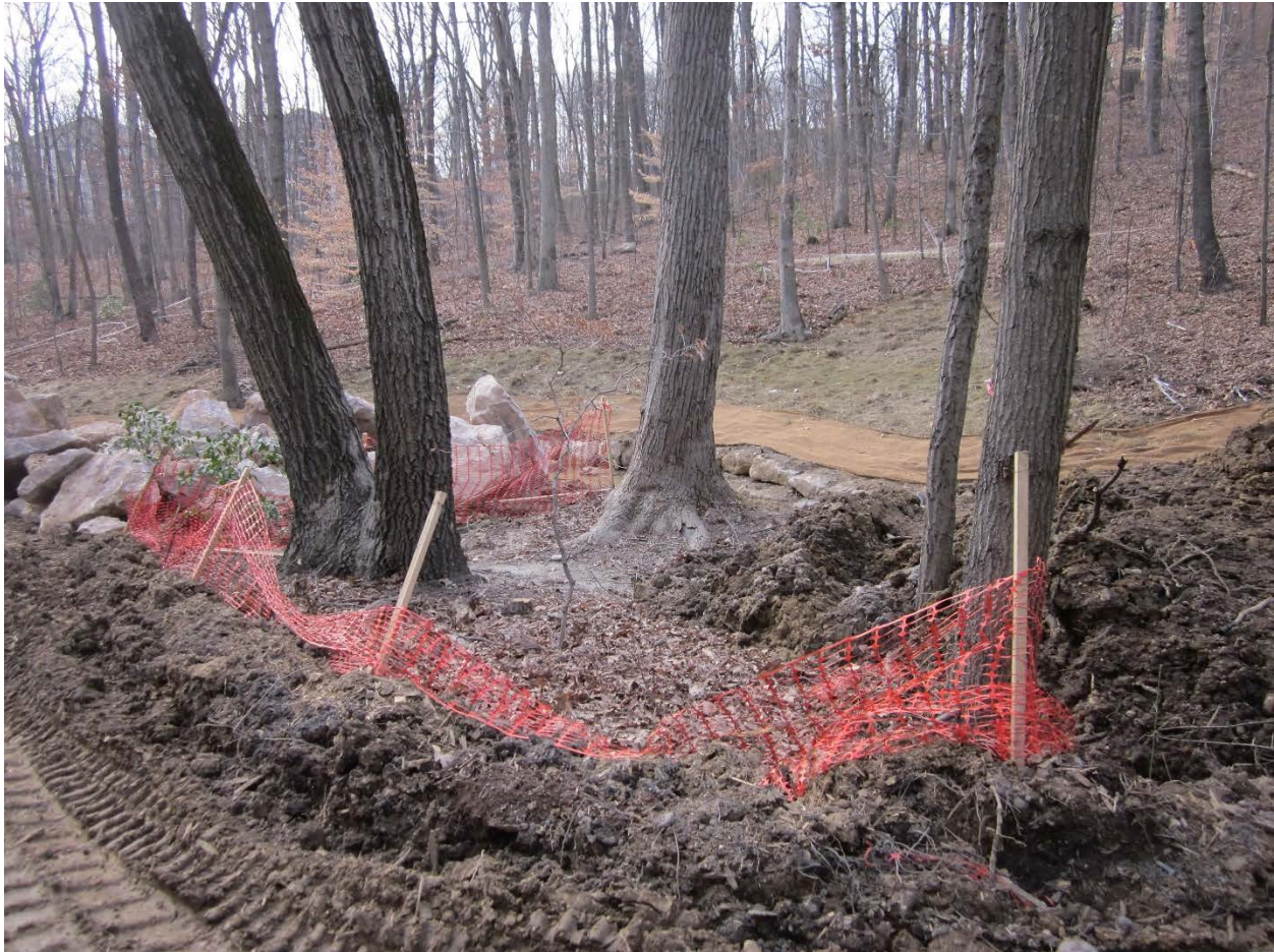
Fig. 3. A “tree save area” within the stream construction project along the upper headwaters of Winkler Run in the City of Alexandria, Virginia. All trees in the save area soon died following construction of the new stream channel as a result of root damage and destruction of the soil microorganisms necessary in sustaining a healthy forest community. This natural channel design project would be considered high-end by many of today’s standards. Photo by R.H. Simmons.
